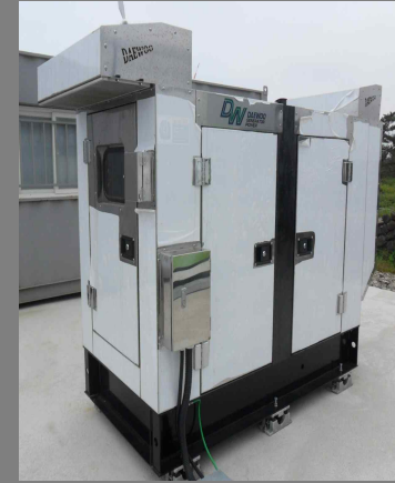
50kW Diesel Generator
