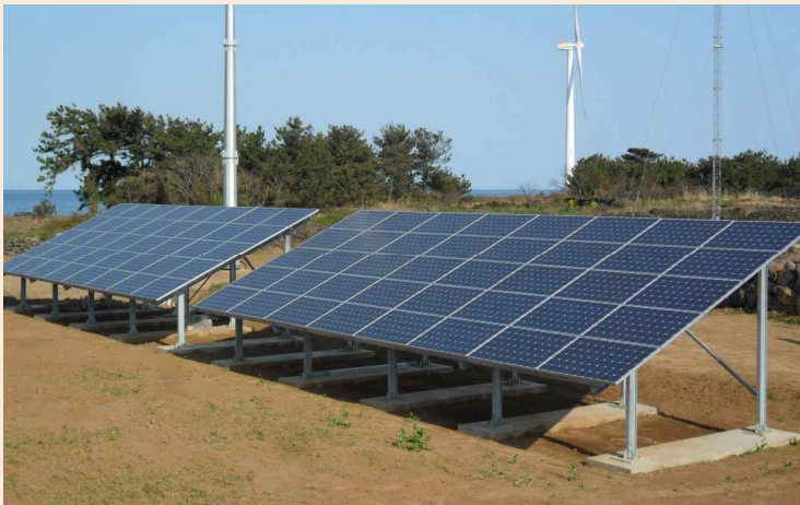
10kW PV Power X2
