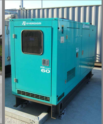
60kW Diesel Generator
