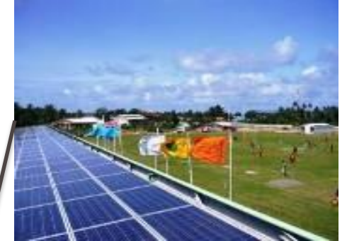
Tuvalu Solar Power Project 40kW. Completed in 2008
